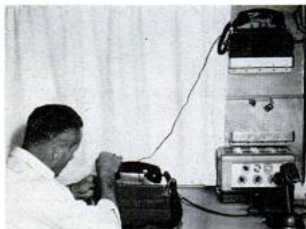
Communication section in front of trailer has two-way radio, portable phones and public-address unit
